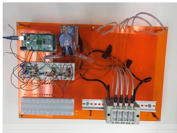
Figure 25: Finalized control system with regulators, RC filter, pump, and Arduino board
