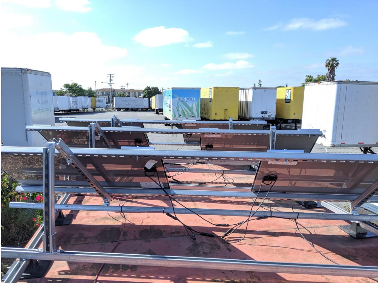
Figure 45. Back view of solar panel system
