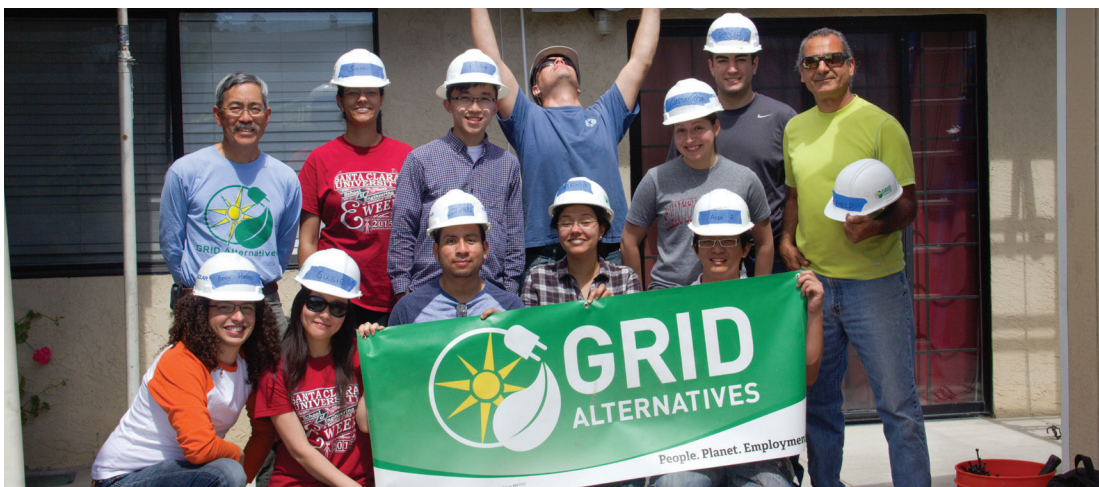
Members of Santa Clara's Energy Club team up with GRID Alternatives to install a residential solar system for a lucky homeowner.
